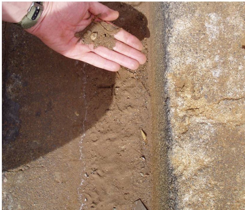
Photo 3 Evidence of Yard-Sourced Contaminants Entering East Street (10/12/04)
