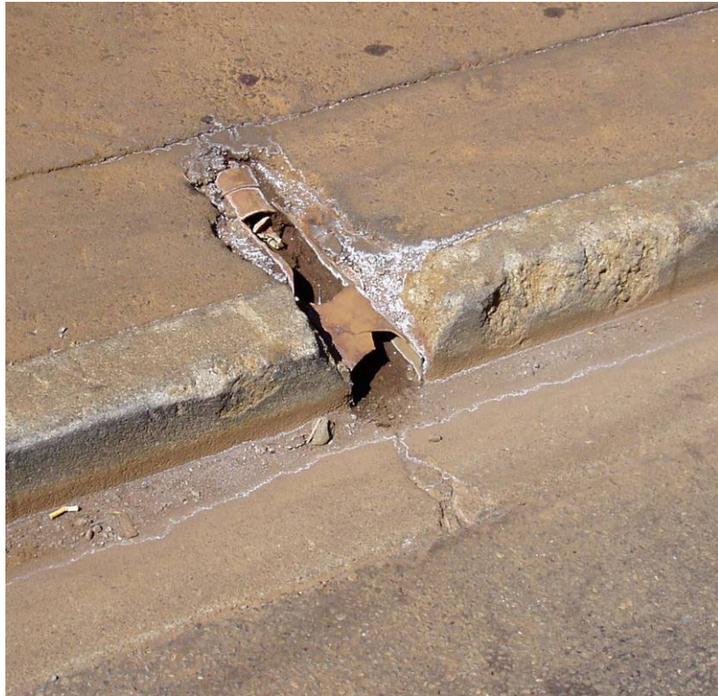
Photo 2 Metallic Debris Accumulated in roadside in East Street (04/11/04)
