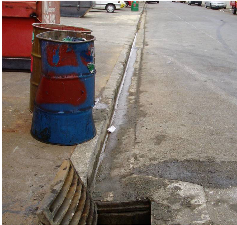
Photo 5 Contaminant Discharge to East Street from Exide Technologies (15/12/05)
