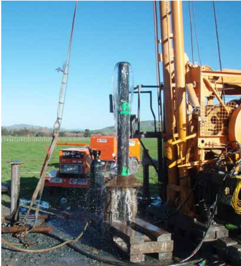
Figure 3.5: Two monitoring boreholes constructed to monitor outflows from the Parkvale area. Note the free flowing artesian groundwater flow from one of the wells.
