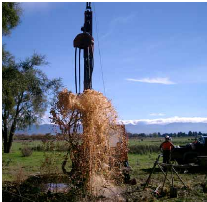
Figure 3.4: Drilling of a monitoring borehole in the Papawai area of the Wairarapa
