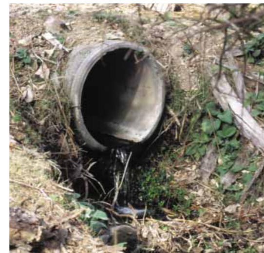
Fish can't migrate up a "perched" culvert
