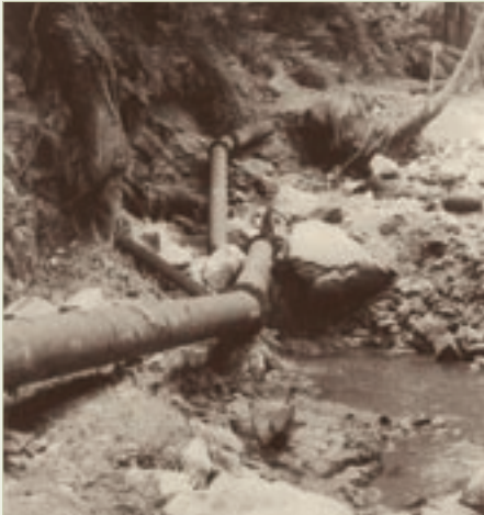
The Boxing Day flood in 1962 resulted in muddy water being supplied to Wellington before the pipe could be shut off.
