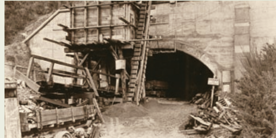
The road tunnel project to link Wainuiomata with the Hutt Valley was abandoned in the 1930s (shown here), but produced dividends when in 1981 it was finished in a smaller bore for water pipes. (Alexander Turnbull Library, Wellington, NZ. Reference F-65767-1/2)
