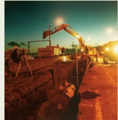
The ‘ten-fifty’ project in the late 1970s greatly increased the supply capacity of the pipeline from Wainuiomata to Wellington.
