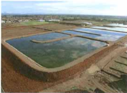
Upgraded Leeston WWTP ponds soon after completion. Infiltration basins are to upper left and border strips are lower right.
