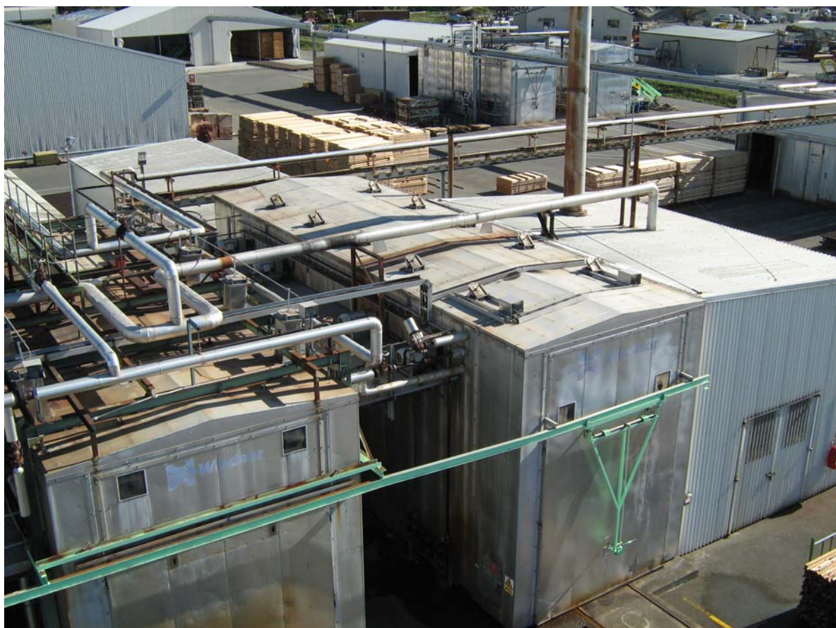
■ Figure 7.2: Photograph of Windsor Kilns 2 and 3 and Oil-fired Boiler Stack
