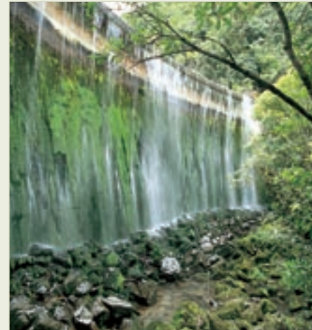
The concrete arch Birchville dam served Upper Hutt for 23 years from 1931, until superseded by the Kaitoke scheme. (Photo Jessica Dewsnap)
