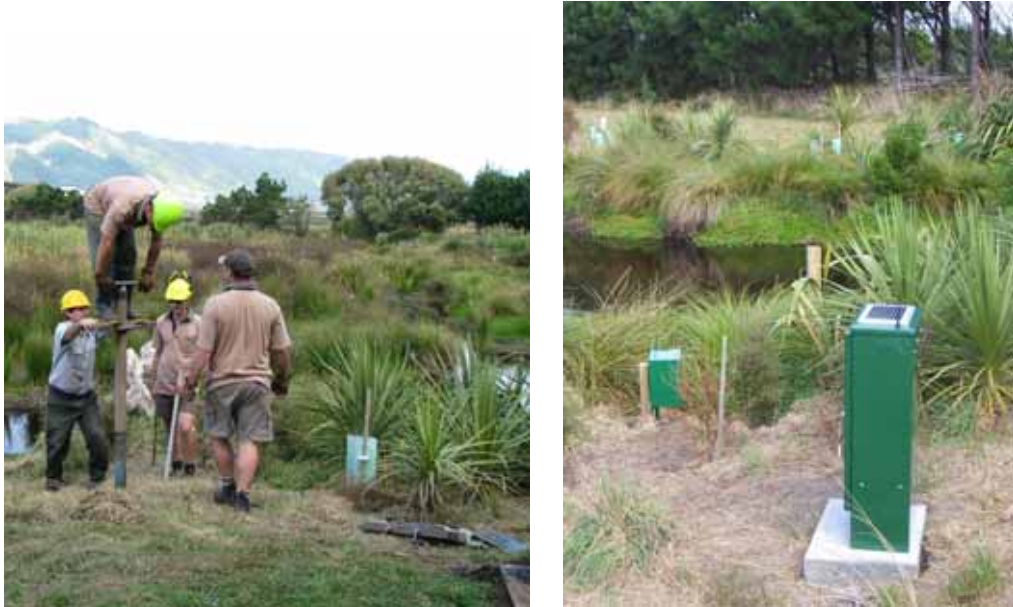
Figure 2.4: Hand-drilling a new borehole next to the Te Hapua wetland on the Kapiti Coast in March 2009 (left) and the final installation, with borehole in the foreground (green box) and wetland staff gauge protruding from open water
