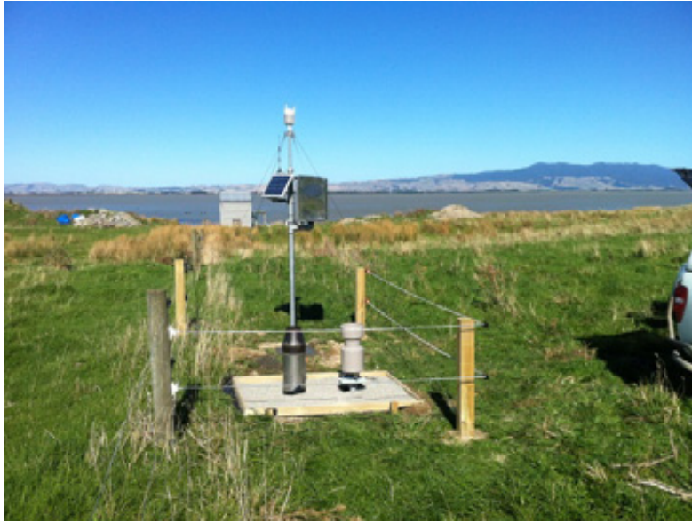
Figure 4.2: Recently installed GWRC met site on the western lake shore (an identical site was installed on the eastern shoreline); instrumentation includes tipping bucket and storage rain gauges, wind speed and direction, solar radiation and air temperature sensors
