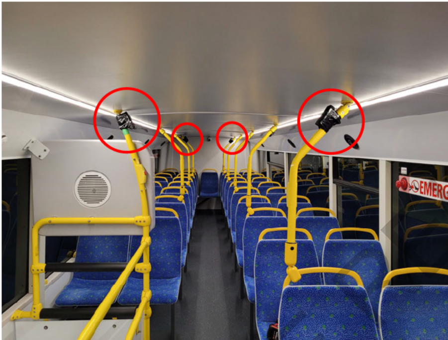
Figure 1. Example of the monitoring installation (red circles) in upper level of Bus 3701.
