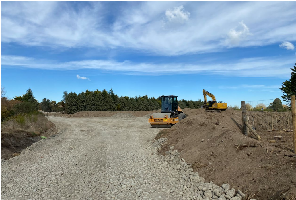
Figure 2: Stage two – Construction of the haul road from the Masterton Recycling Centre through to the Ruamāhanga River
