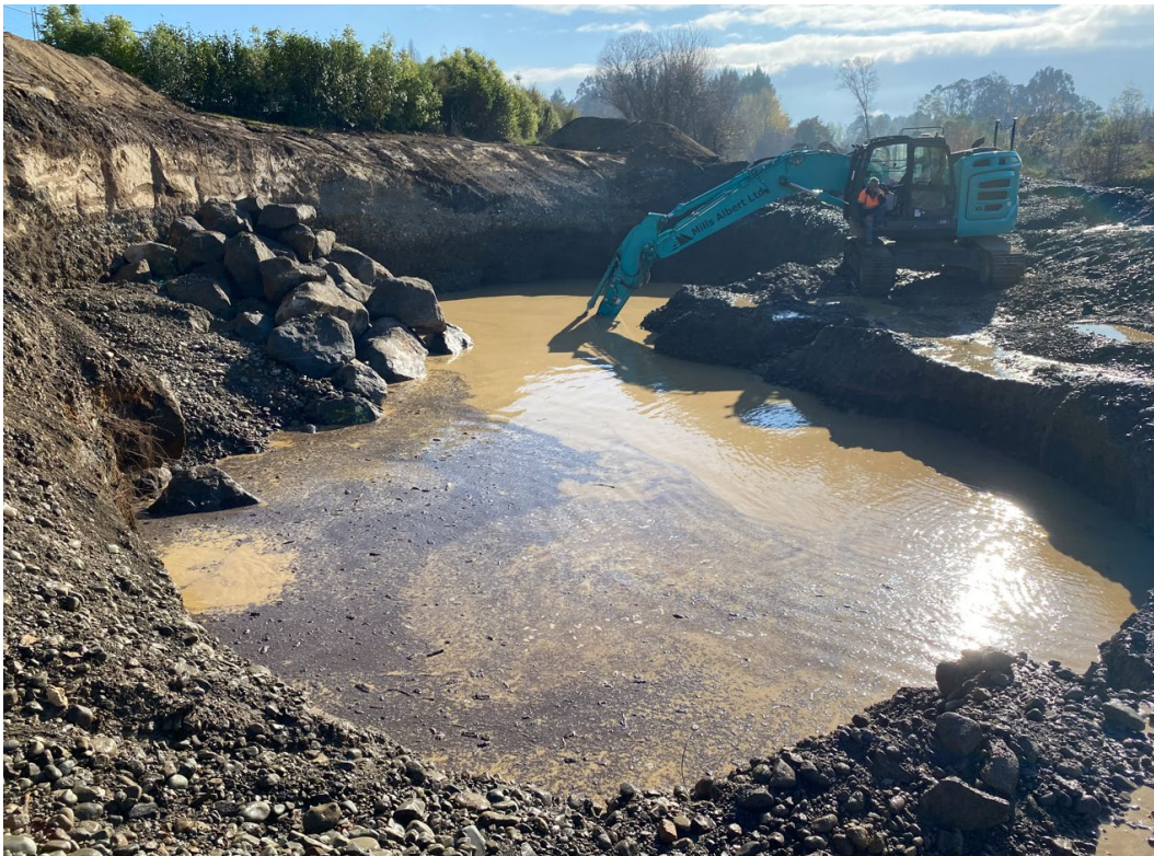
Figure 4: Stage two (Waipoua River) – Excavation of the rock groyne within the Waipoua River (the excavation is bunded from the Waipoua River and is not within the flow of the river)
