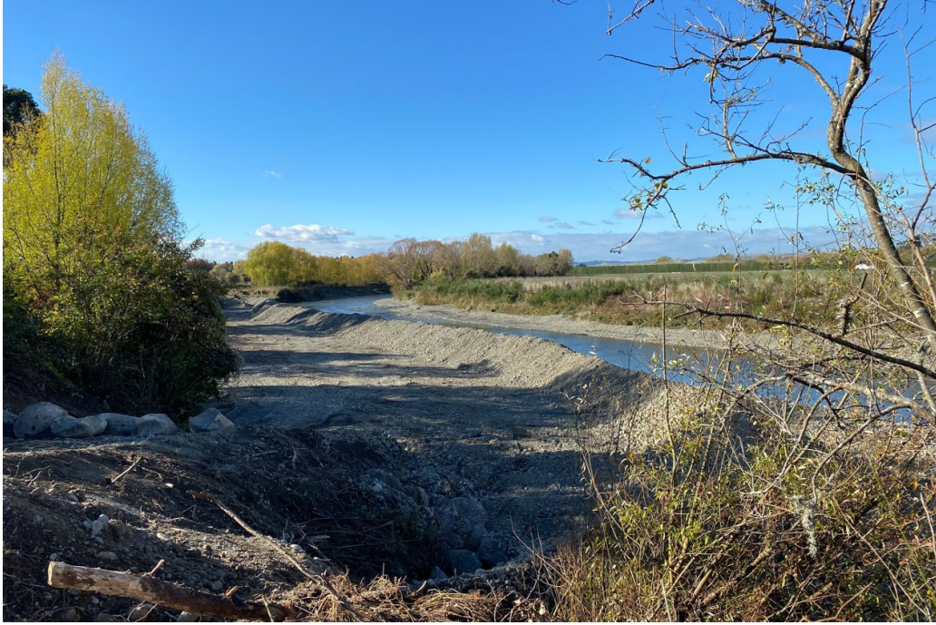
Figure 1: Stage two (Ruamāhanga River) – Temporary river diversion, temporary beach and bunding complete
