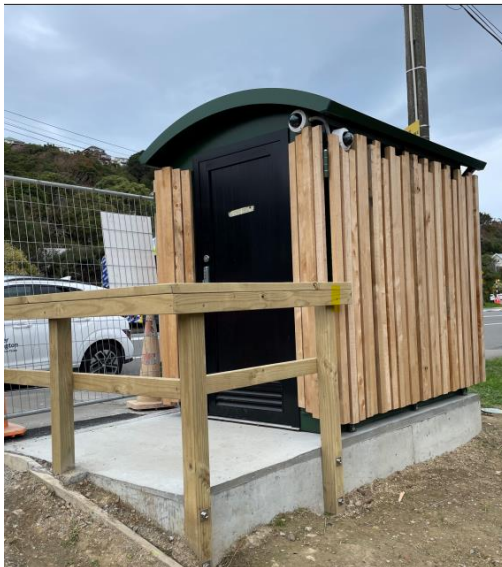
Image 3: Facility – installation completed – photo prior to opening (Karori)
