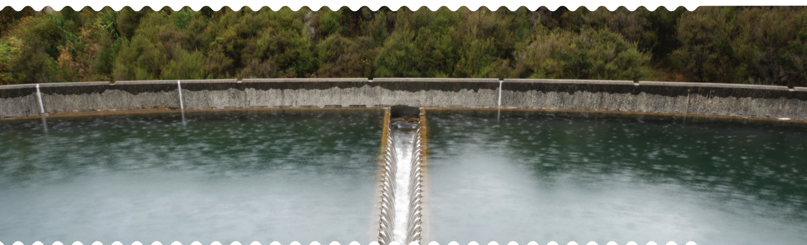
A clarifier at Greater Wellington's Te Mārua drinking water treatment plant.
