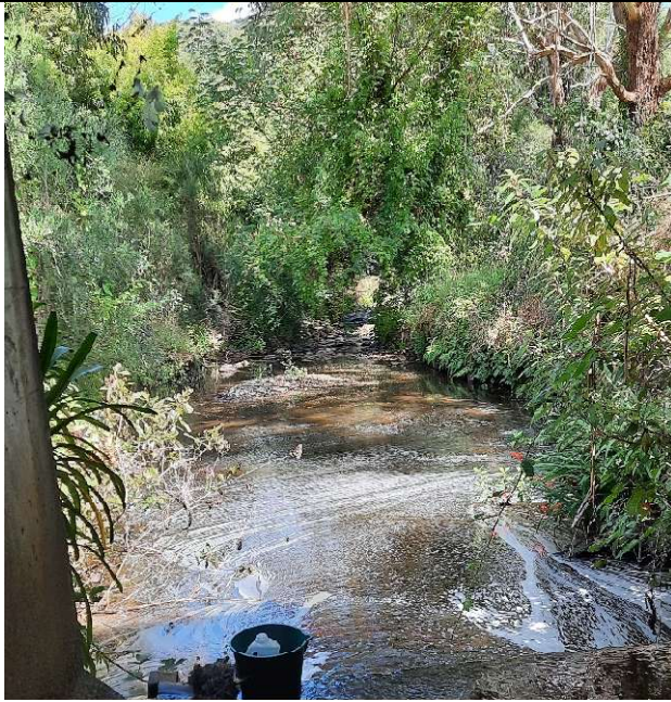
Caption: Blaikies stream outlet viewed from inside culvert, Fairly low VC as listed in Table 1
